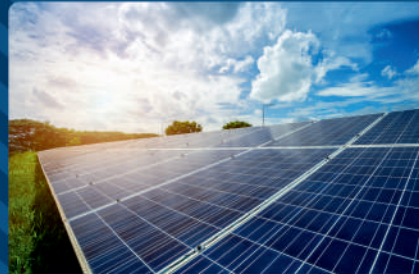
Solar Panel System
